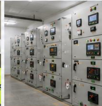
VCB PANELS & HT SWITCHGEAR
